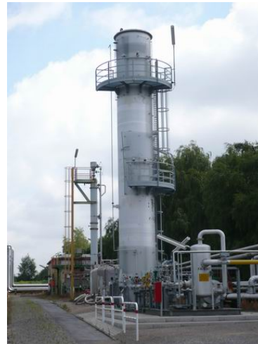
Complete combustor unit.
